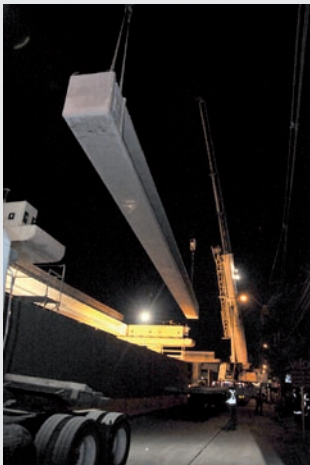
» Placement of the first beam of the viaduct of the new Line 5 stretch.
